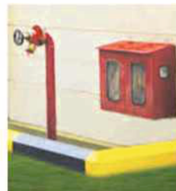
REFERENCE IMAGE FOR FIRE HYDRANT
